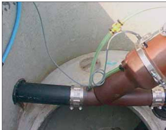
Valve monitoring transmitter installed on Iseki RediVac Interface Valve
