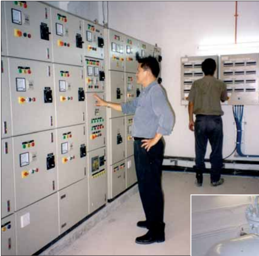
Motor Control Centre complete with integral PLC and valve monitoring console
