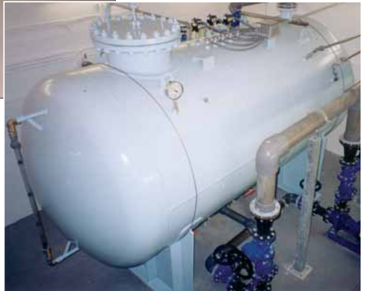
Steel sewage collection vessel
