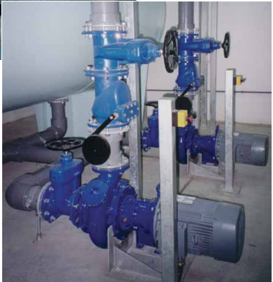
Dry well, centrifugal screw sewage discharge pumps
