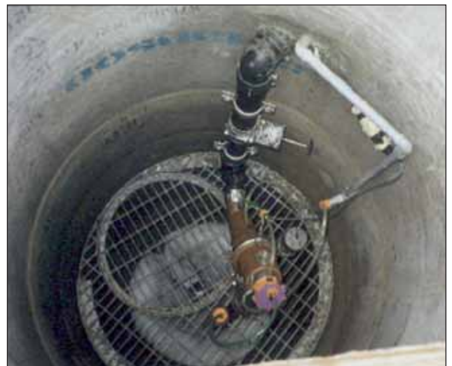
Valve chamber fitted with high level warning equipment.
