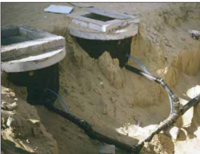
Connection of collection chambers to valve monitoring system
